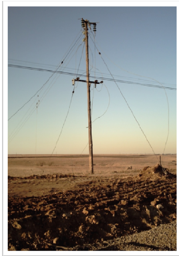
Figure 2 showing severed electrical power cables.
