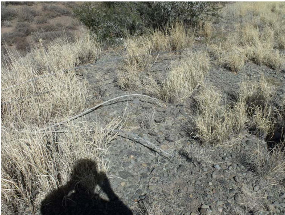
Figure 3. The severed power cable.
