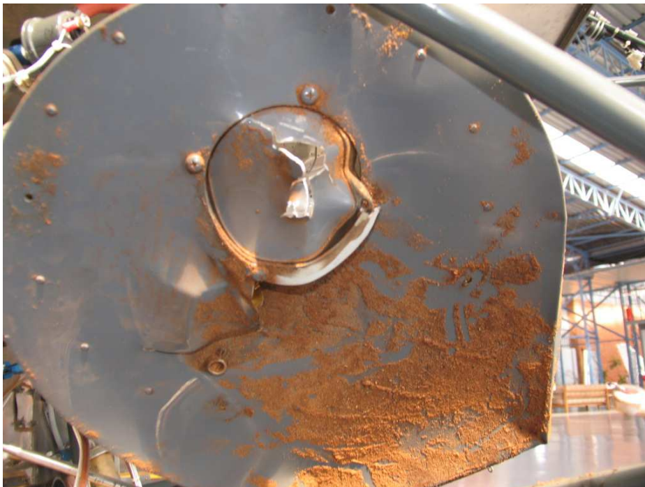
Figure 6. A view of the lower section of the air filter box which was in contact with the sand.
