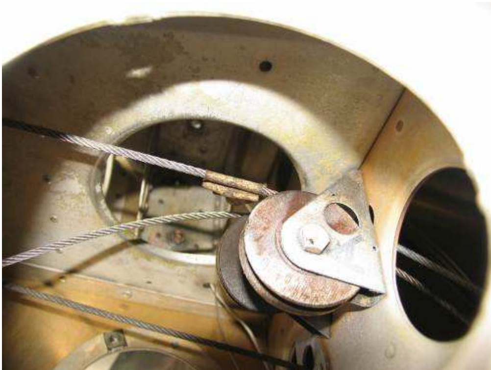
Figure 8. Photo of the rudder cables and pulleys taken through the inspection panel (maintenance in progress)
