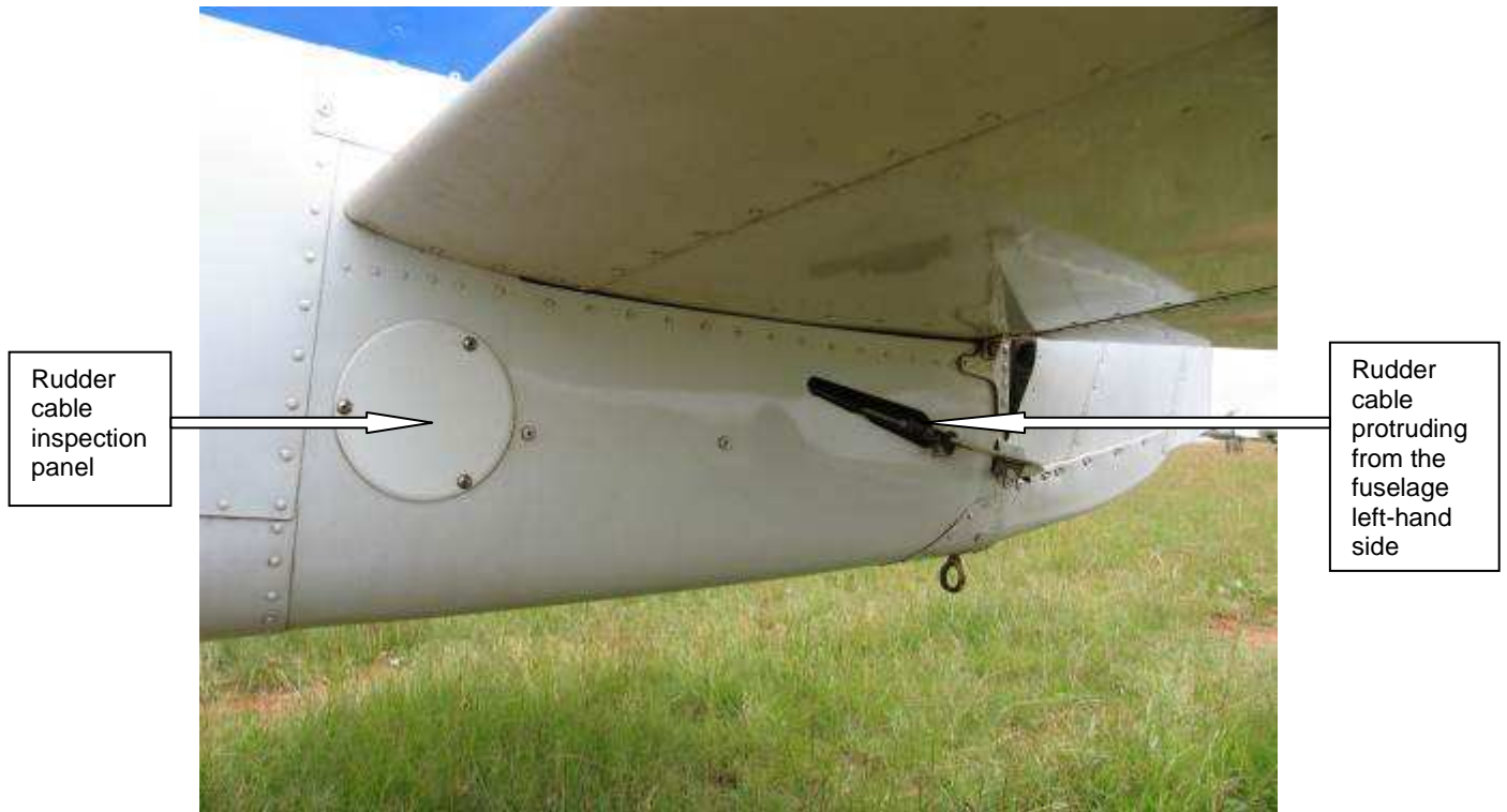
Figure 6. A view of the inspection panel as well as the rudder cable and attachment bracket
