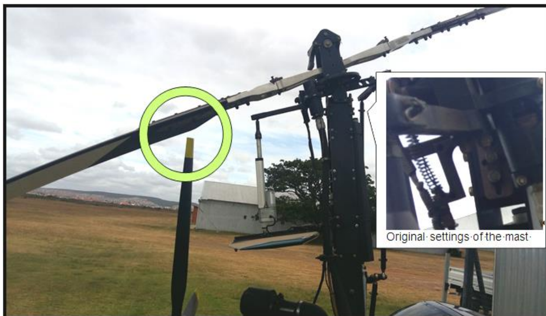
Figure 9: Shows the clearance with the original adjustment as it was found on the aircraft type
